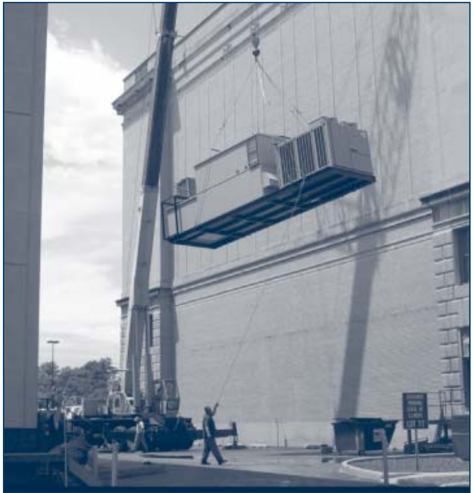
A 9-ton dehumidification unit was hoisted onto the roof of the Margaret Cross Norton Building on the Capitol Complex in Springfield on July 18, 2003. The addition of the unit is part of an ongoing project to provide a new, environmentally sound heating, venting and air-conditioning system for the building's multi-layered record storage areas.
